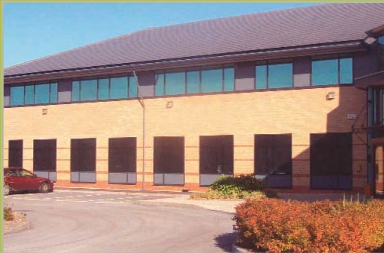
Crime Shield screens fitted to lower office windows to provide vandal and glass protection. HS Shoreshield type
